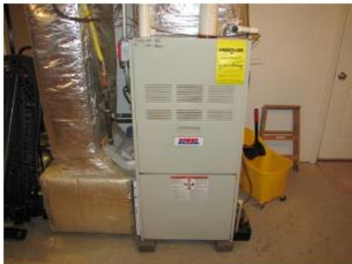
HEIL forced air, oil fired furnace
