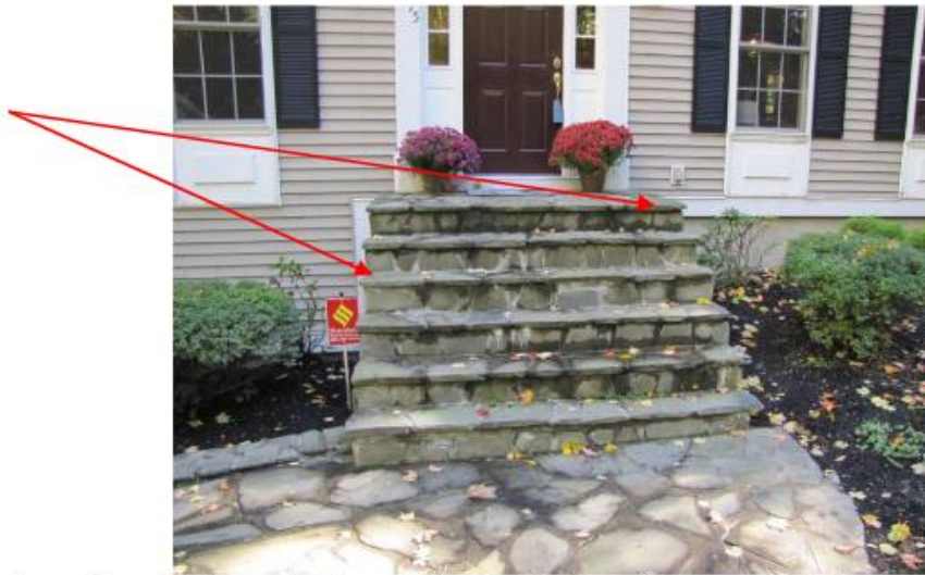
Front porch and steps missing safety handrail system and showing minor deterioration
