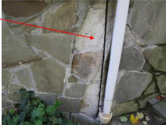
Stone veneer wall covering falling off of home
