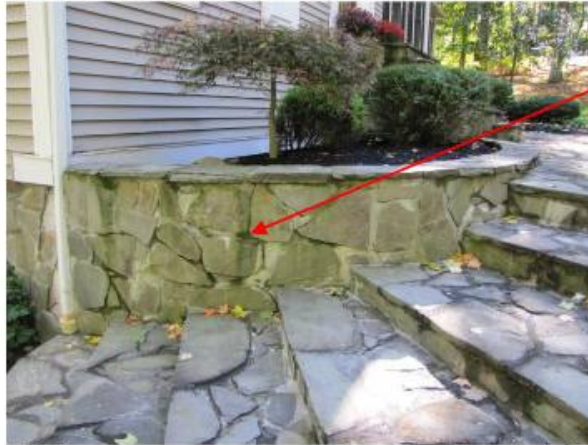
Stone retaining wall showing some signs of mortar joint deterioration and failure
