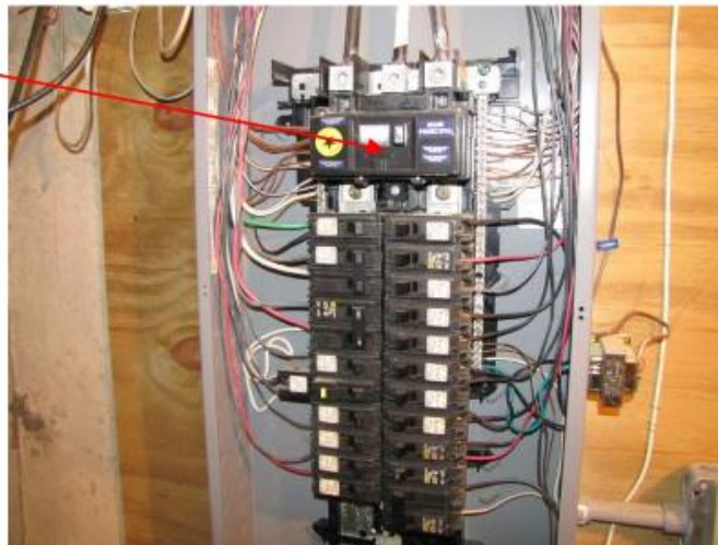
Main electrical panel showing main disconnect
