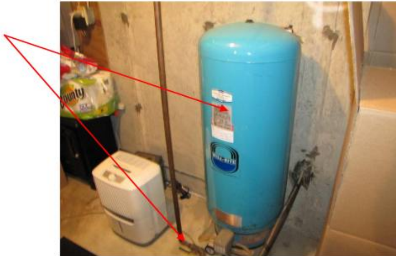
Well water bladder tank showing main shutoff valve
