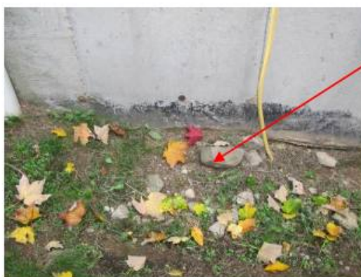
Apparent rainwater ground erosion
