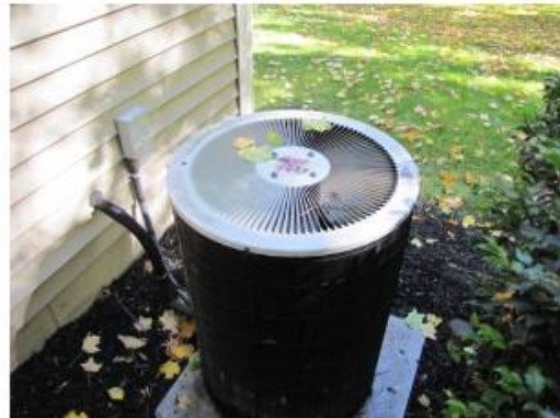
Matching HEIL A/C condensing unit
